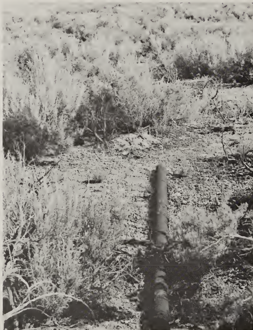
Figure 36: Sections of the water pipeline leading from the reservoir to Terrace can be seen in the desert. Looking southwest towards Terrace Mountain. (BLM photo)
